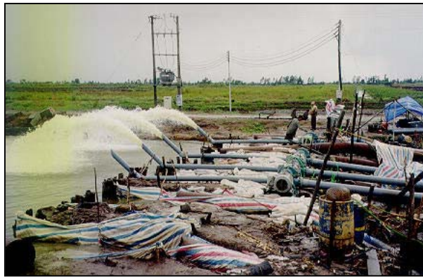
Figure 8. Salt water pumped into canal system for fire control
